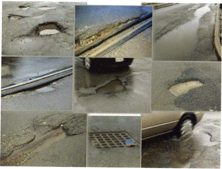
FIGURE A.2: Photos of the identified “potholes”, including some false positives Source: Pothole Patrol (2007)
