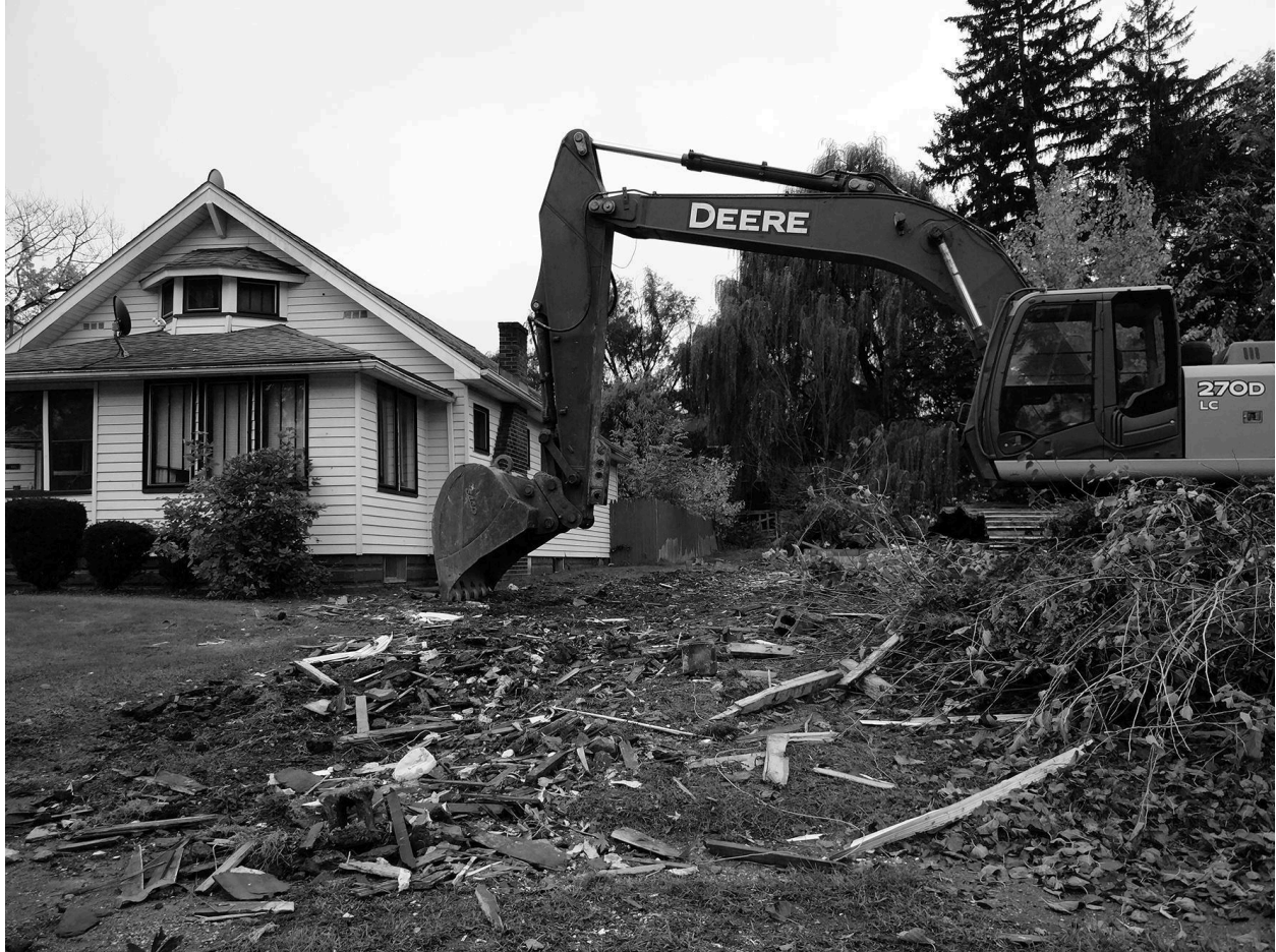
Figure 3. Demolition is widespread in Youngstown. The single-family house formerly occupying this site in a Youngstown neighborhood was demolished in October 2017. Photograph by authors.
