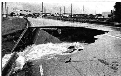
(a) Flooded Roads
