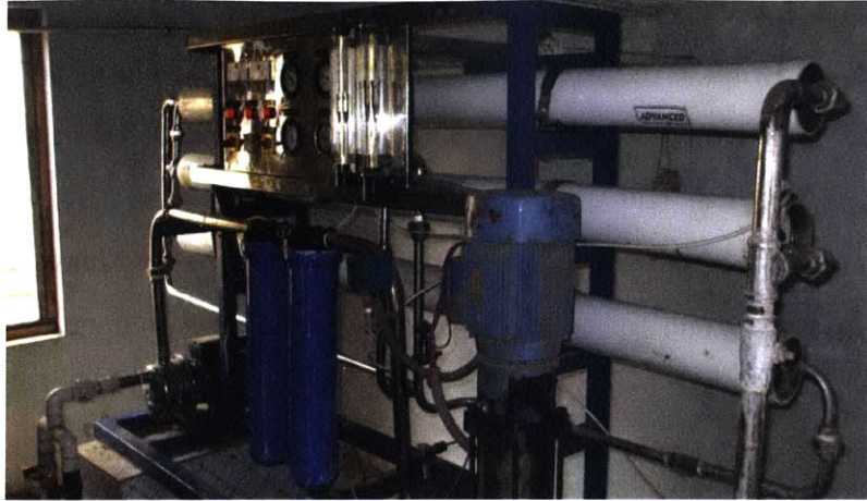
Figure 1-5: Tata Projects, based in Hyderabad India, has installed approximately 3000 reverse osmosis system (shown here) and ultrafiltration plants across India.
